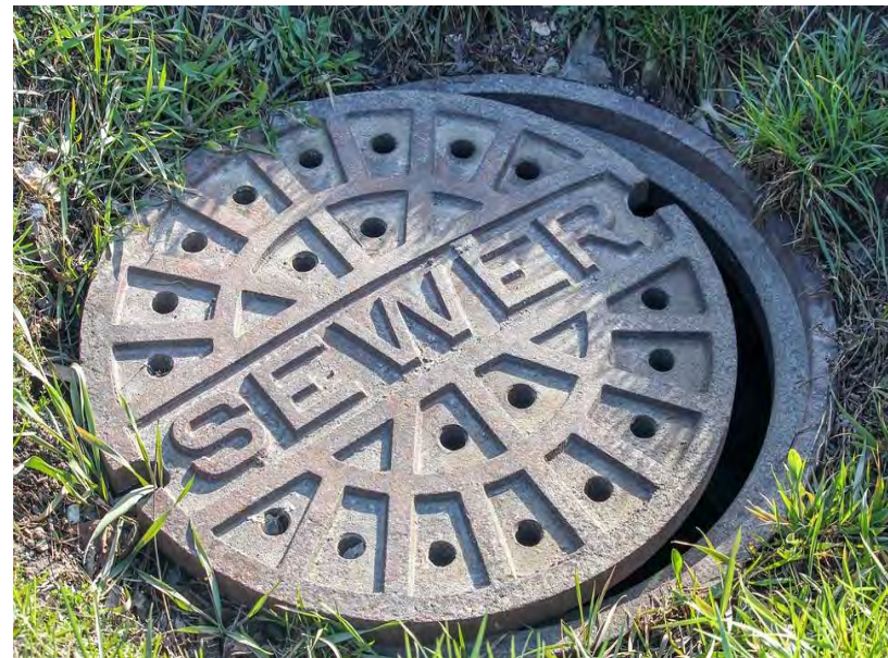
Figure 30. Sewer manhole cover (Pixabay).
