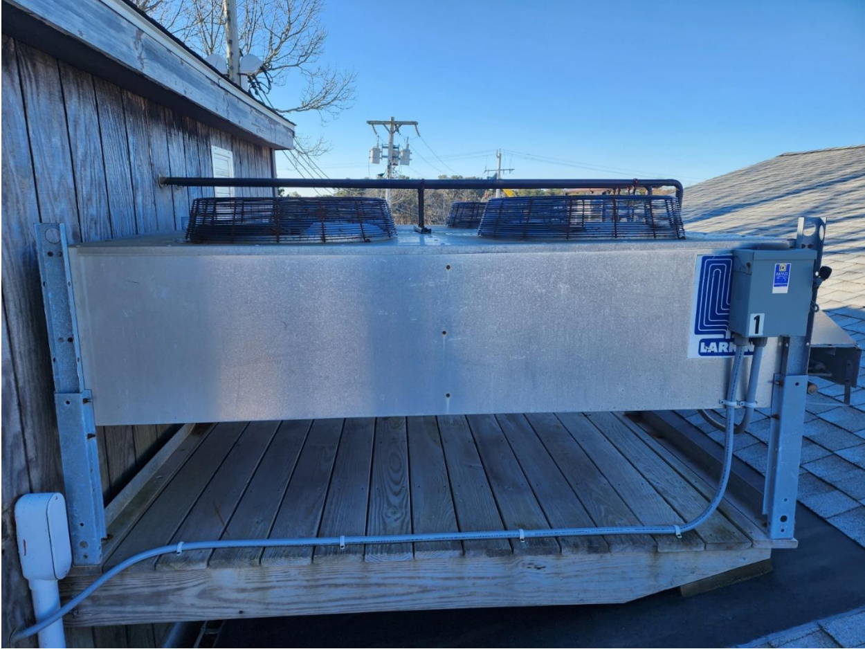
Figure 6 Close up of Condensing Unit
