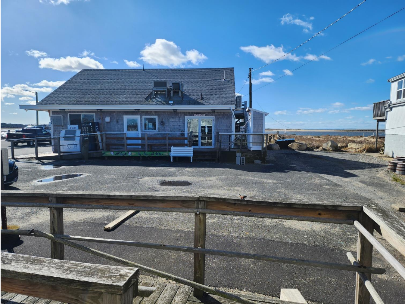
Figure 2 Proposed site looking south. Note the asphalt patches for existing underground utilities running to the South and to the East
