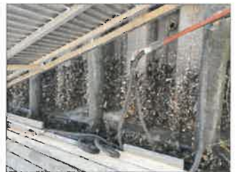
8. FUEL LINES TRANSITIONING FROM GANGWAY TO FLOATING DOCK
