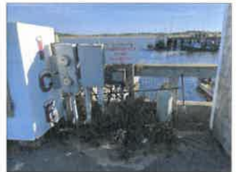
4. EMERGENCY SHUTOFF SWITCH
