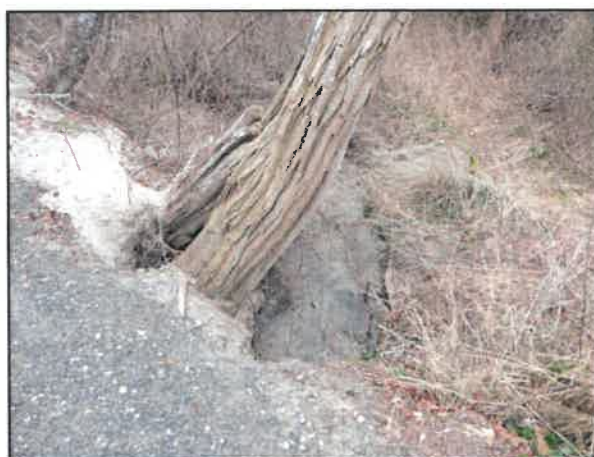
Road erosion into Herring River at Old Kings Highway crossing ( J. Portnoy 2019 )
