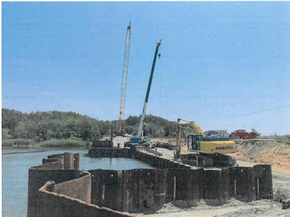
Figure 4. – View looking south across the river. Showing temporary bridge abutments, and stone armor coffer cell.
