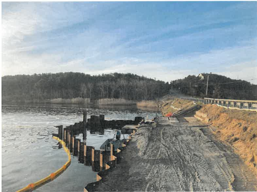
Figure 2. – Showing steel sheet coffer cell where MIG installed 5' thick stone armor for scour protection.
