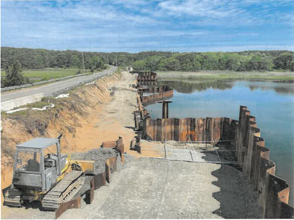
Figure 3. – View looking north across the river. Showing temporary bridge abutments with steel tie-rods, and stone armor coffer cell.
