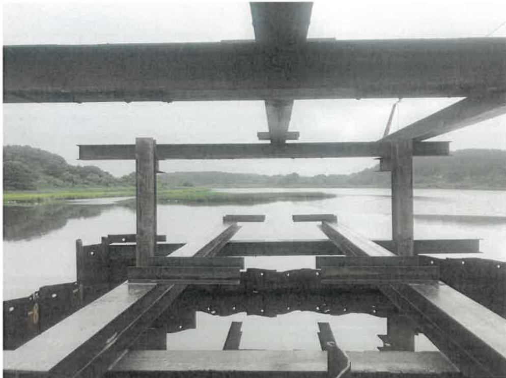
Figure 6. – View showing false work installed in anticipation of temporary bridge pile installation.
