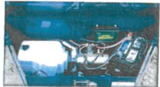
Pump & battery box, w/ optional battery tender
