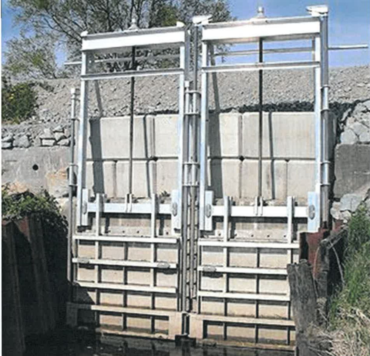
Figure 5. Example of an adjustable tide gate (Golden Harvest GH-50) that would meet Mayo Creek tidal-restoration and infrastructure-protection objectives, based on hydrodynamic modeling (Woods Hole Group 2016). Such a design would allow the Town complete control of the opening to ensure that water levels meet social and environmental
