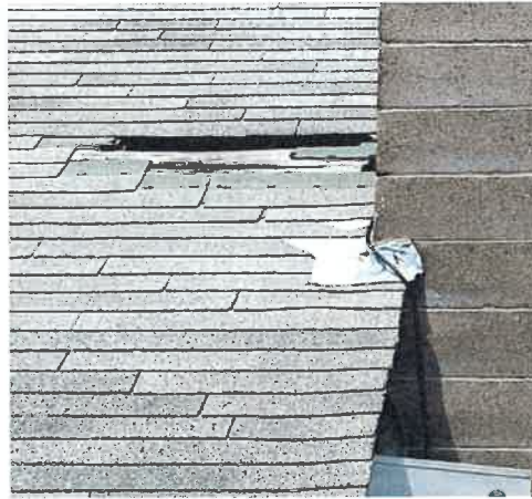
Missing shingles, Hole?
