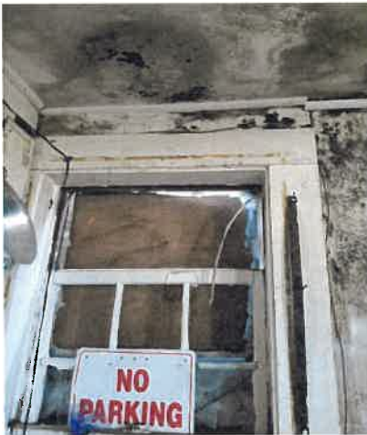
Broken Windows, Mold Thraughtout.
